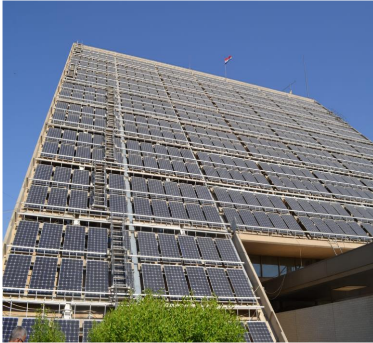
Figure (2): The 135kW REERC PV system.
