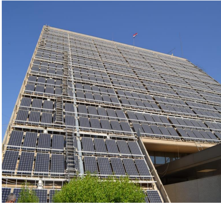
Figure (2): The 135kW REERC PV system.
